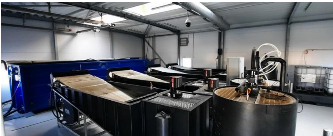
Figure 4 Flocculation and mechanical separation cleaning system
